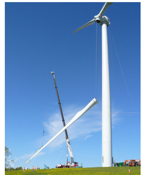
Cheap blade repair Clipper’s new method uses a winch and two industrial trucks
